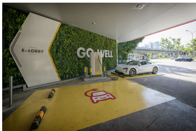
An electric vehicle (EV) charging bay at a Shell service station in Singapore is one of many popping up around the country as EVs become more popular, and better supported through policies and infrastructure. | Photo: Bryan van der Beek/Bloomberg via Getty Images
