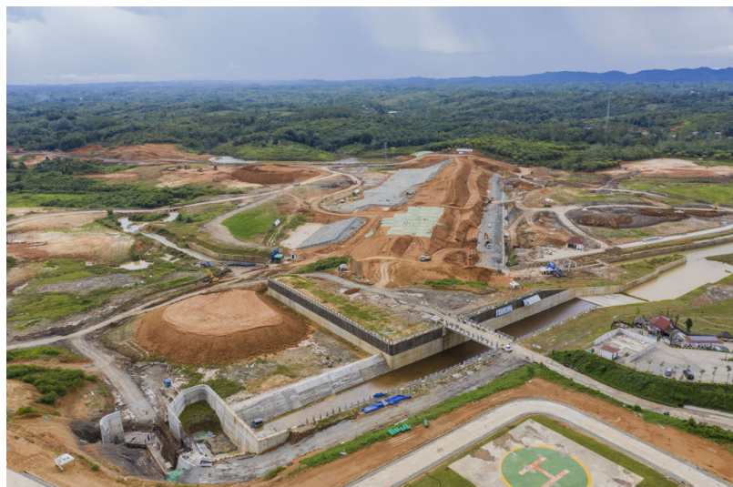
Sepaku Semoi Dam under construction at the country’s new capital Nusantara, known as IKN, in Penajam Paser Utara, East Kalimantan province, Indonesia, Wednesday, March 8, 2023. Indonesia is offering more tax cuts and looser terms for land acquisitions under a new rule as it seeks to attract more investors to its US$34-billion new capital project. | Photo: Rony Zakaria/Bloomberg via Getty Images
