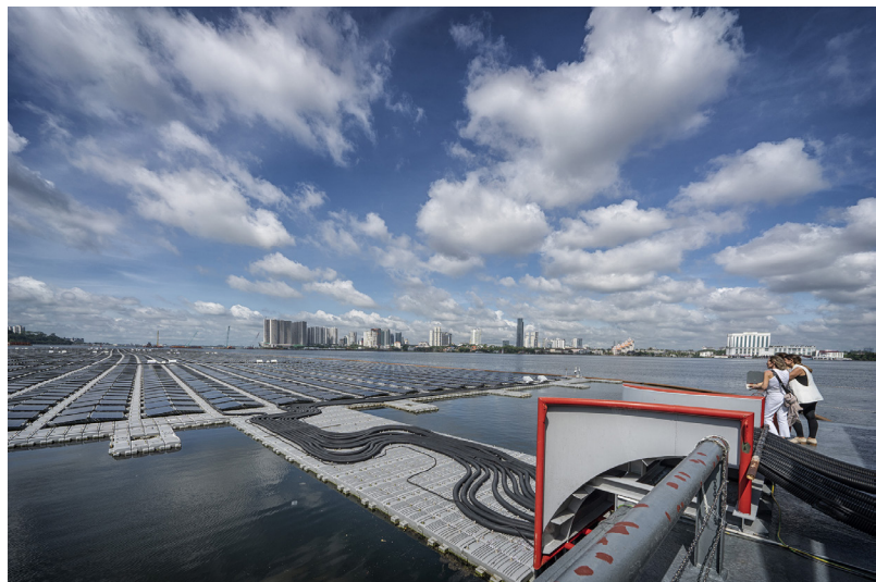
This floating solar photovoltaic power plant by EDPR Sunseap Group, a unit of Energias de Portugal SA, in Woodlands, Singapore, supplies power to the national grid. | Photo: Bryan van der Beek/Bloomberg via Getty Images
